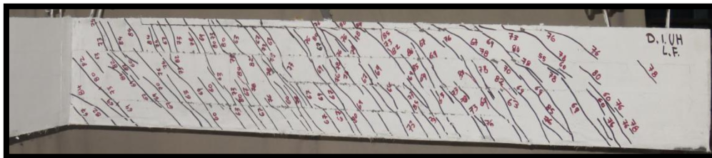
Fig-13: Crack pattern of beam D-1-UH at failure
