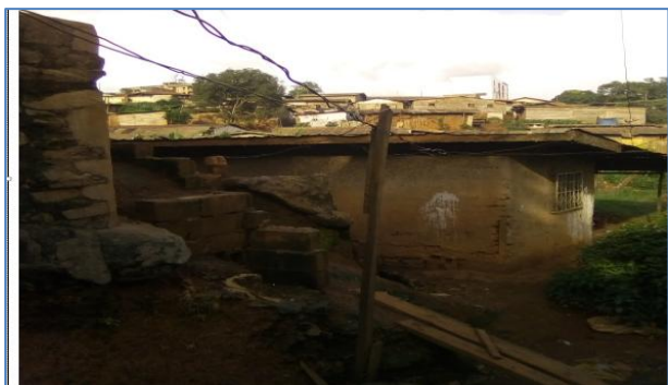
Photo-1: Unorthodox Distribution of Electrical Energy in the Azegue Neighborhood
